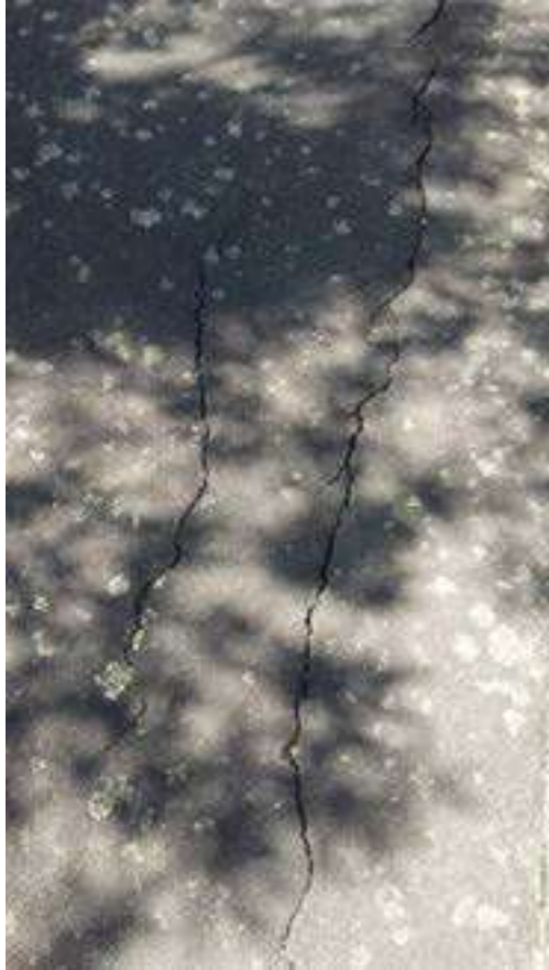
Cracked asphalt on entrance footpath
