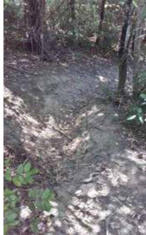
Washed out gravel path and blocked drain
