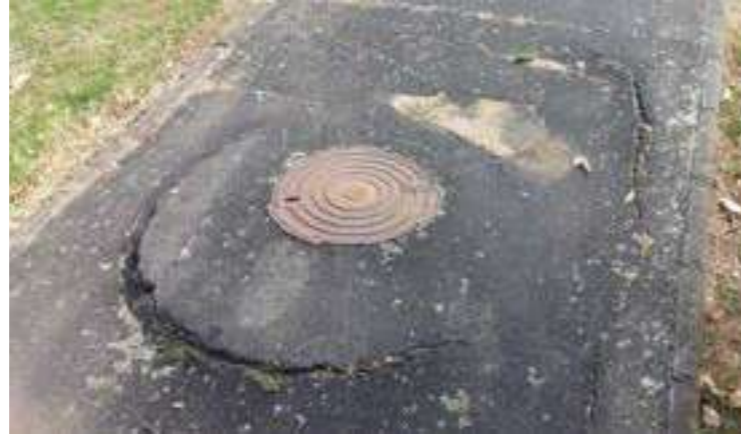
Exposed manhole on asphalt footpath creating a trip hazard
