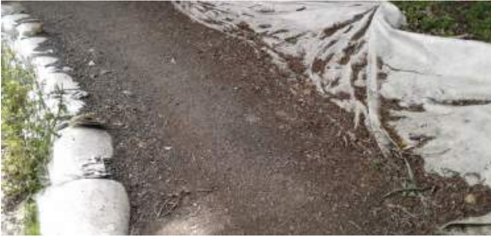
Figure 21: Temporary path remedial work in Ōrākei Basin East, awaiting the upgrade project
