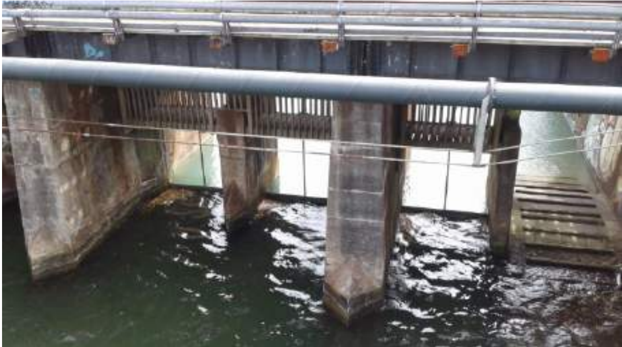
Figure 26: Sluice gates programmed for upgrade to an automated operation
